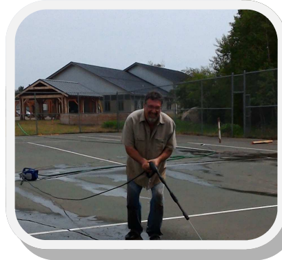
Marc Smith pressure washing the cracks on the tennis court in preparation for patching
